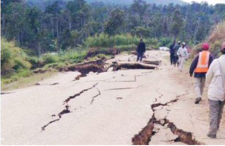
Damaged road in Komo, Hela province of Papua New Guinea, affected by the 7.5 earthquake 26 February 2018. Photo - Radio New Zealand
